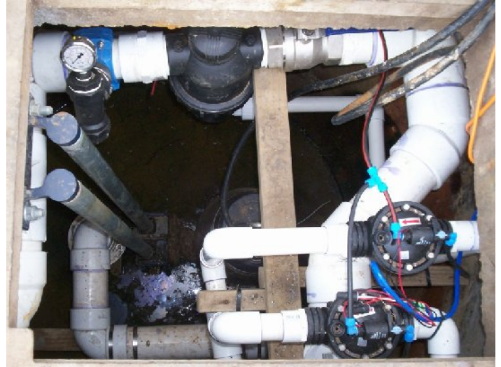
The new pump installed in the underground pump house.
