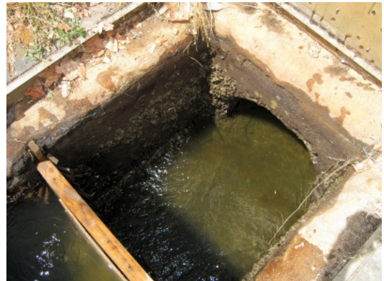
The weir gate chamber, the leak is alongside the exit pipe top centre in the photo.
